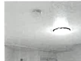
Smoke/Carbon Monoxide Detector inside guest room 2
