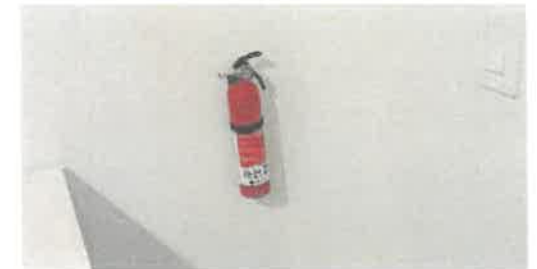
Fire Extinguisher – entry of guest bedroom/bath kitchenette area
