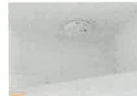
Smoke/Carbon Monoxide Detector inside guest room 1
