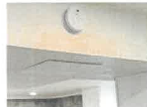
Smoke/Carbon Monoxide Detector outside bathroom and guest room 1
