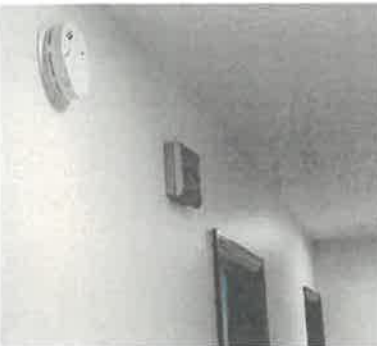
Smoke/Carbon Monoxide Detector outside of guest rooms
