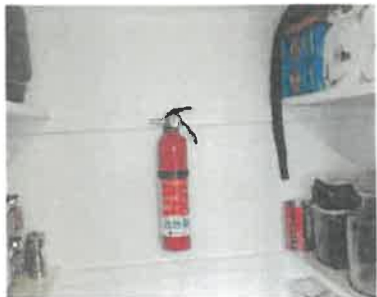
Fire Extinguisher in kitchen pantry – 7 ft from stove
